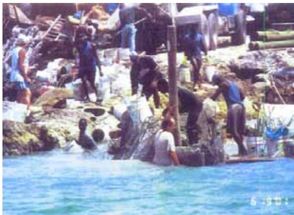
Unauthorised and destructive construction of artificial reef on Nygard Property
