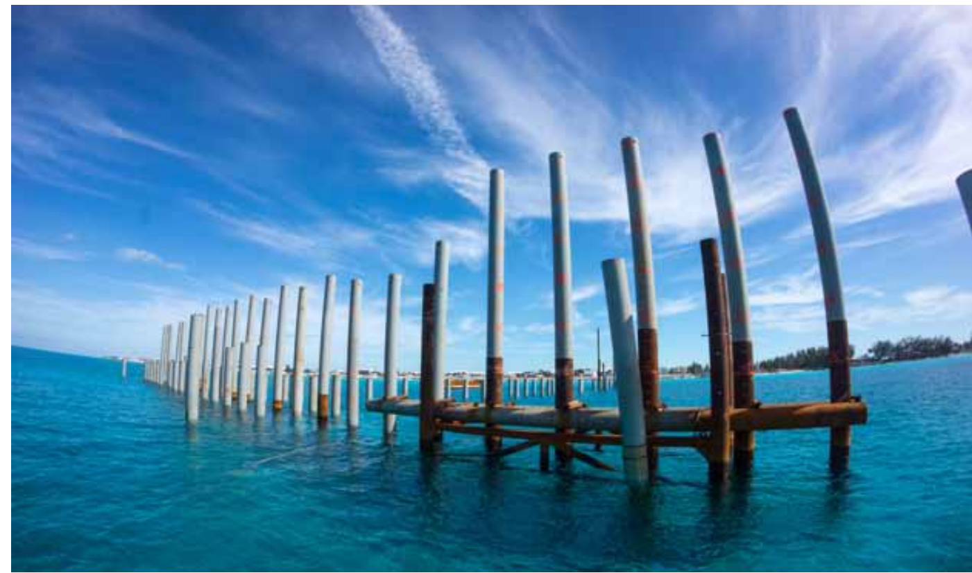
Pilings driven into the seabed off North Bimini as part of the preliminary work for Resorts World's controversial 1,000 foot pier and accompanying 4.5 acre docking "island".
