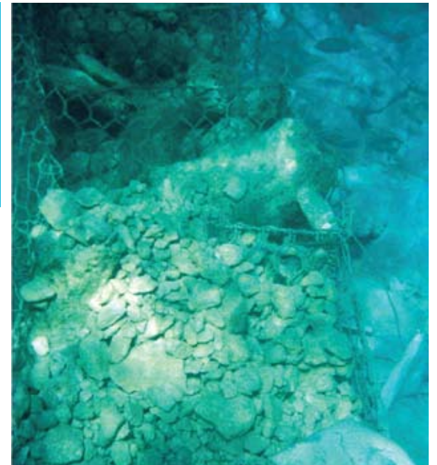
“Most of the gabions were broken up, and there was a substantial amount of rock debris” (2011 University of Miami Report).
